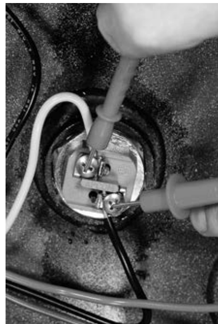
Figure 19. Element Voltage Test
